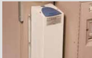
Uninterruptible Power Supply (UPS)
